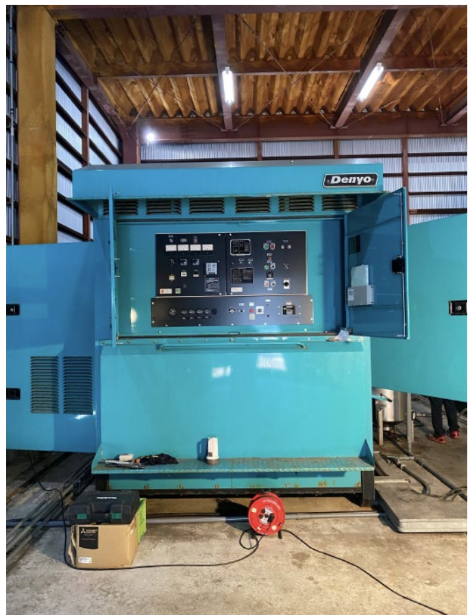
Diesel Electricity Generator
